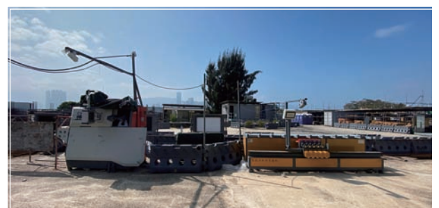
Computerised automatic bar-bending and cutting machines
