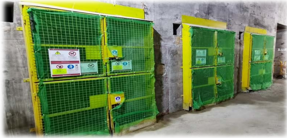
Lift shaft were covered with safety nets to prevent any falling objects
