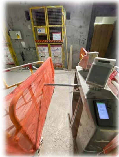
Lift shaft Permit-to-work system
