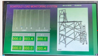
(monitoring system at site office)
