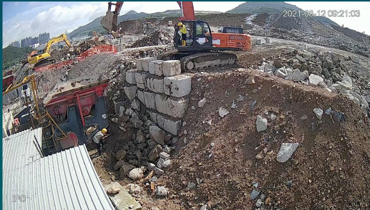
(1) Worker enter danger area under excavation
