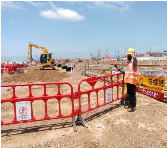
Red Barrier for Fatal Zone Identification
