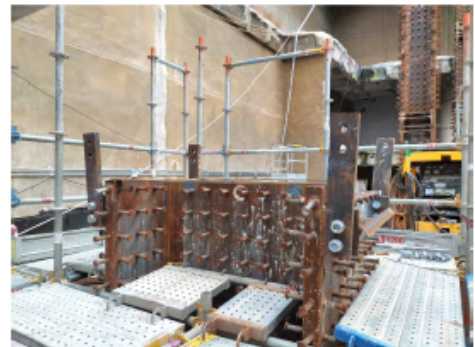
CHECK BEFORE ERECTION
