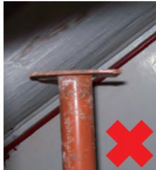
Props Do not Support The Ceiling
