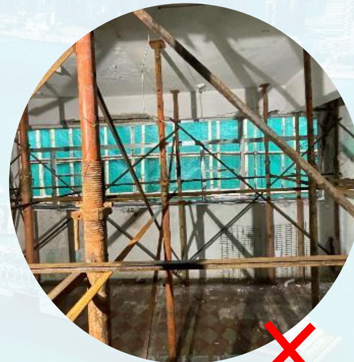
Props not erected in accordance with the approved plans
