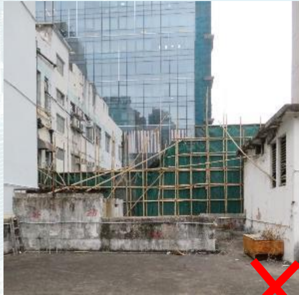
CCTV not provided in accordance with the approved demolition plans
