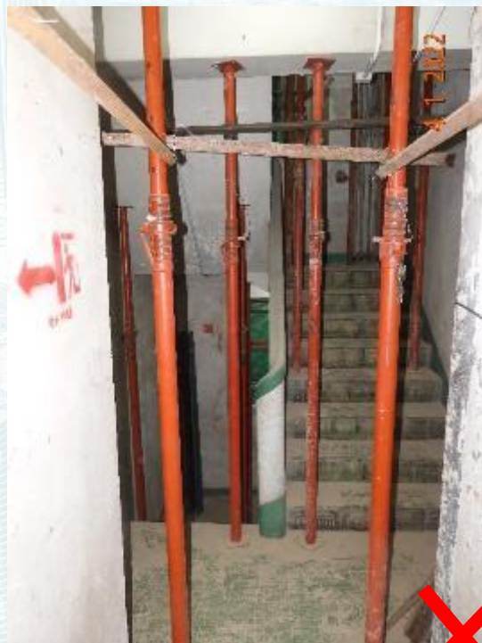
Inadequate bracing to the propping
