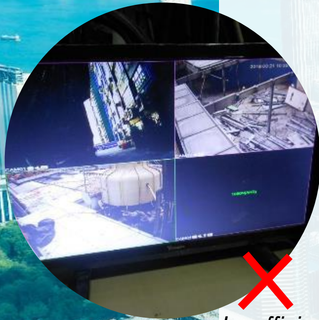
Insufficient coverage of CCTV
