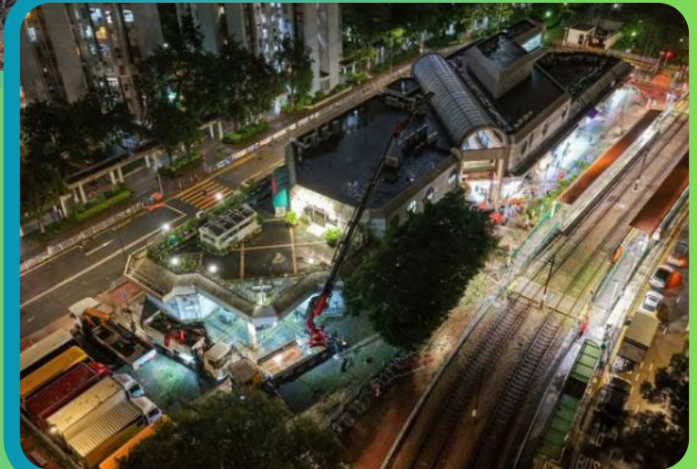
↓ Emergency Response to Fallen Trees onto LRT railway and power cable due to Typhoon
