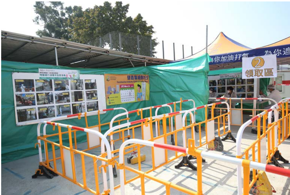
The Kai Tak Sports Park site located at Muk Tai Street participates in the Construction Industry COVID-19 Testing Day
