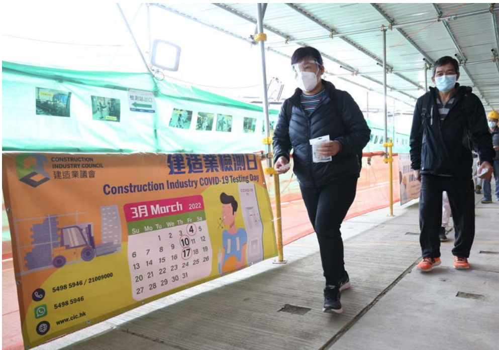
After receiving the Rapid Antigen Test (RAT) kits, workers enter the construction site in separate groups
