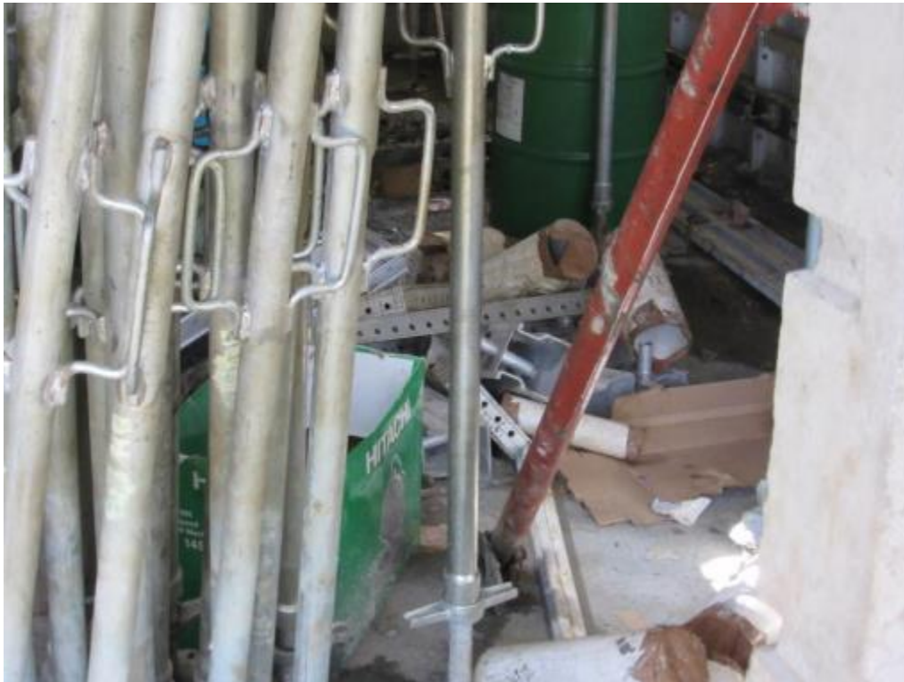
Photo 53: Construction Wastes Noted in the Working area of Aluminium System Formwork
