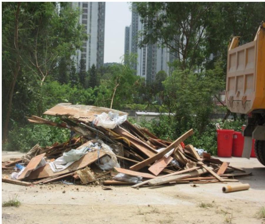
Photo A5: Debris from Site C (I)
