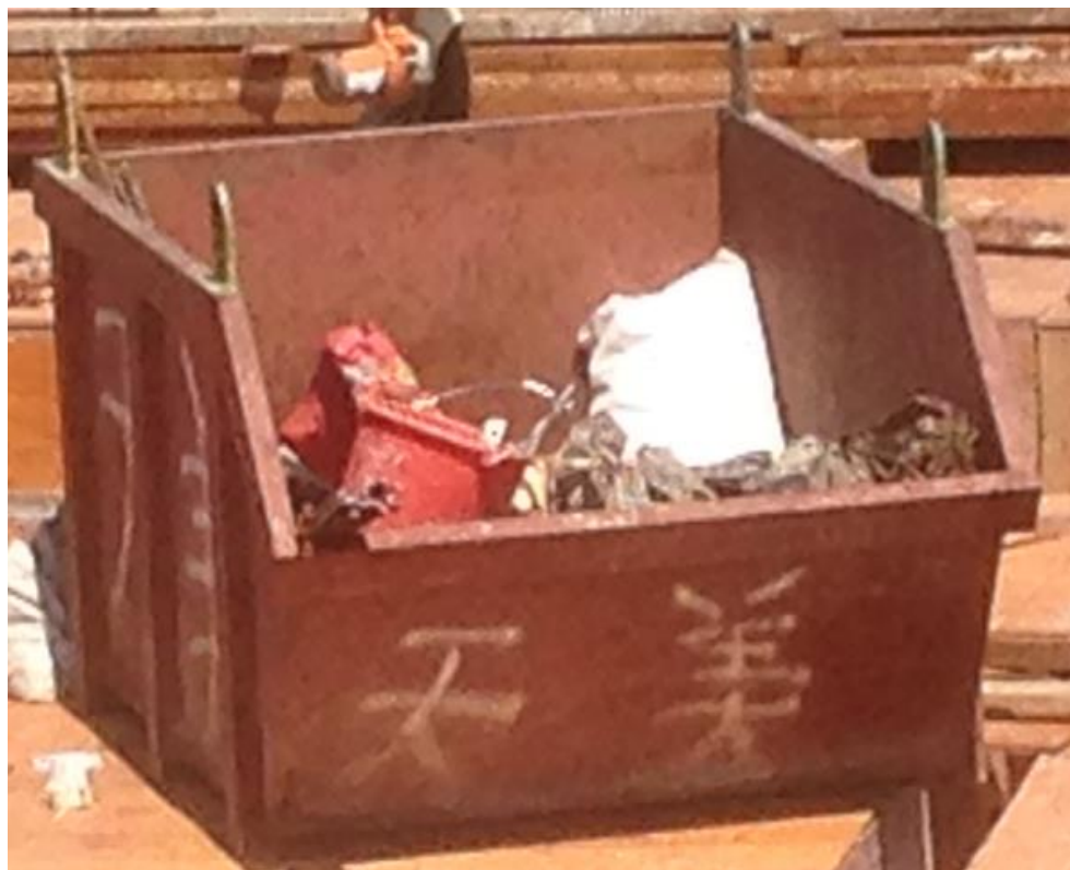
Photo 90: Small Skip for Collecting Waste at the Working Area (2)
