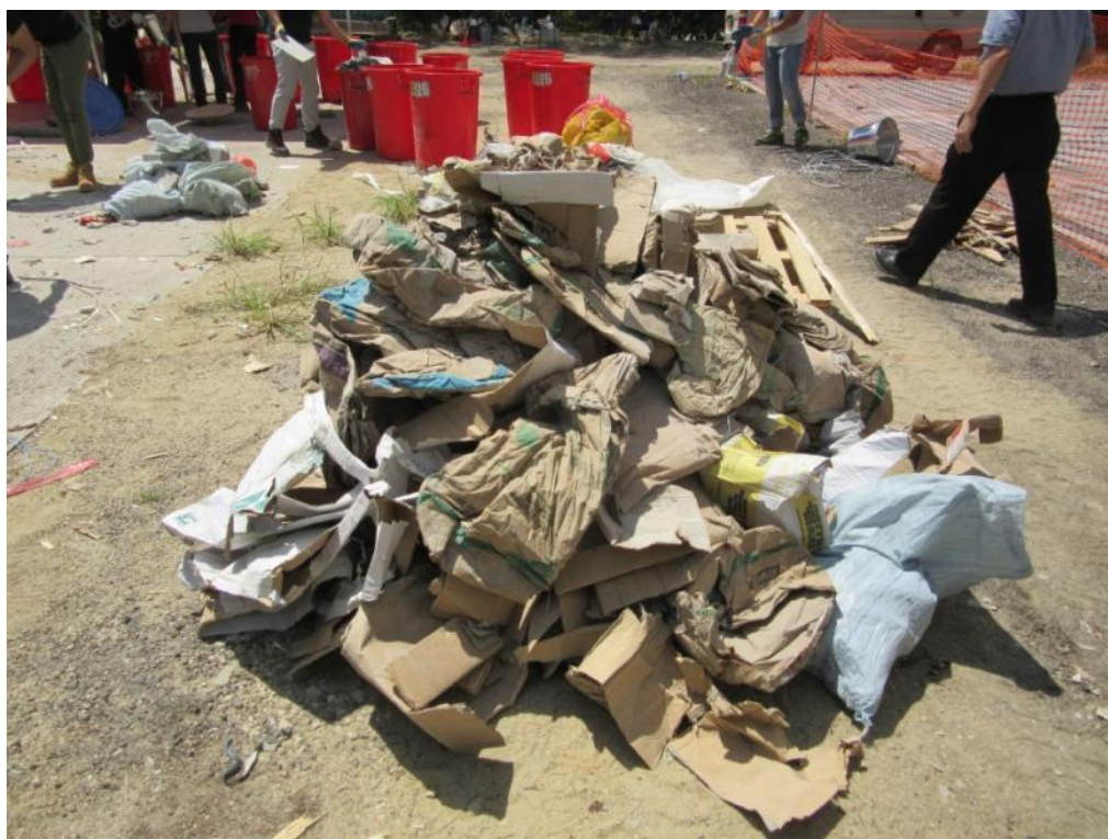
Photo A24: Some Other Construction Waste from Site A (II)
