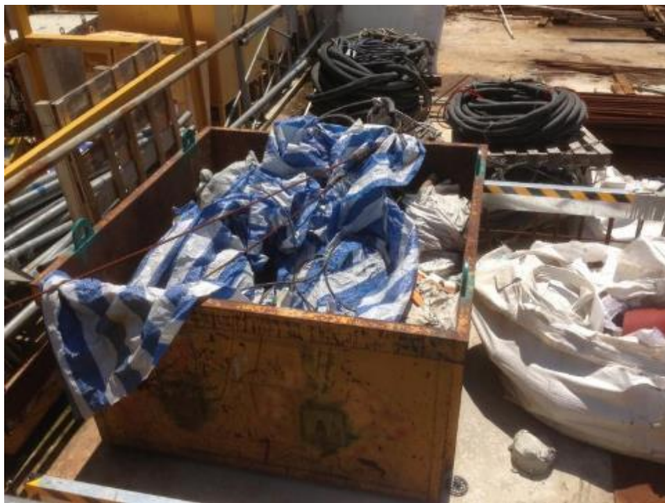
Photo 83: Contents of Construction Waste in Skip A (Mainly Consisting of Nylon Canvas, Steel Bar & Cable etc.)
