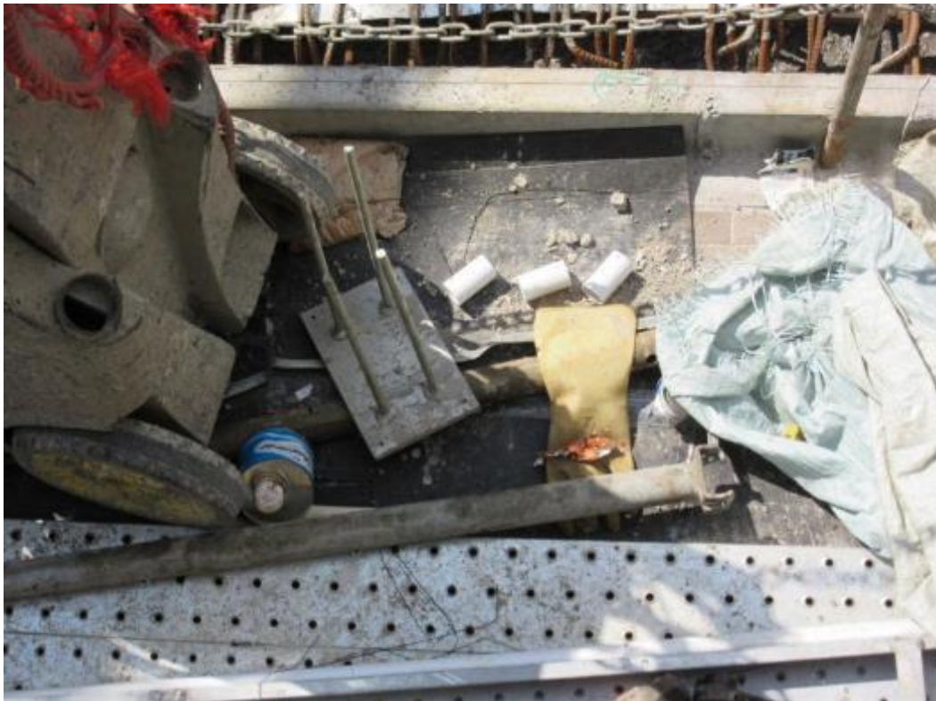
Photo 52: Construction Wastes Noted Near to Concreting Area
