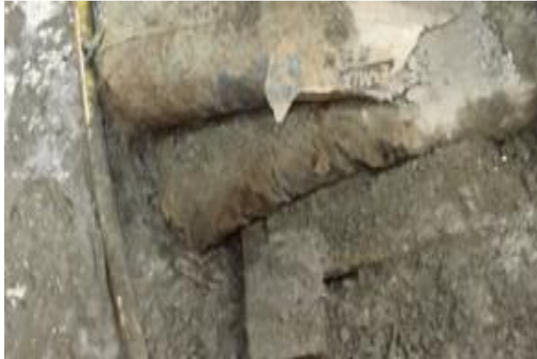
Photo 21: Damaged Bolding Agent due to Water
