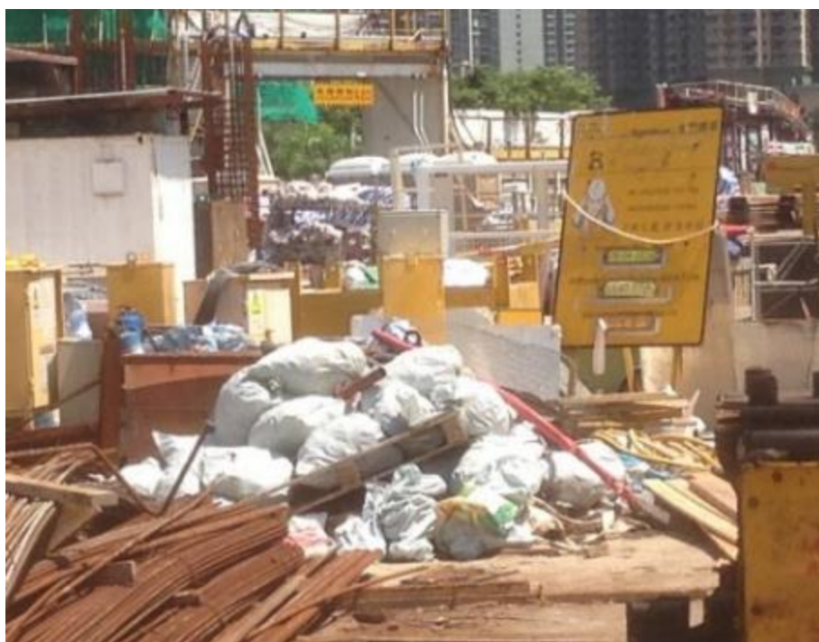
Photo 86: Contents at a Temporary Dumping Location (Mainly Consisting of Timber Pallet, Cable, nylon bags and Steel Scraps etc.)
