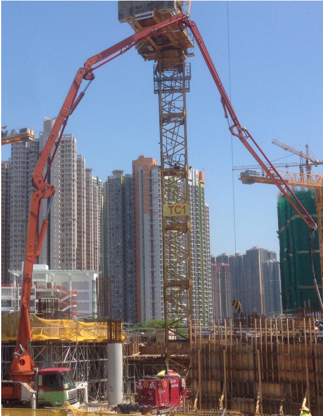
Photo 78: Pipe System of Concrete Pumping Machine
