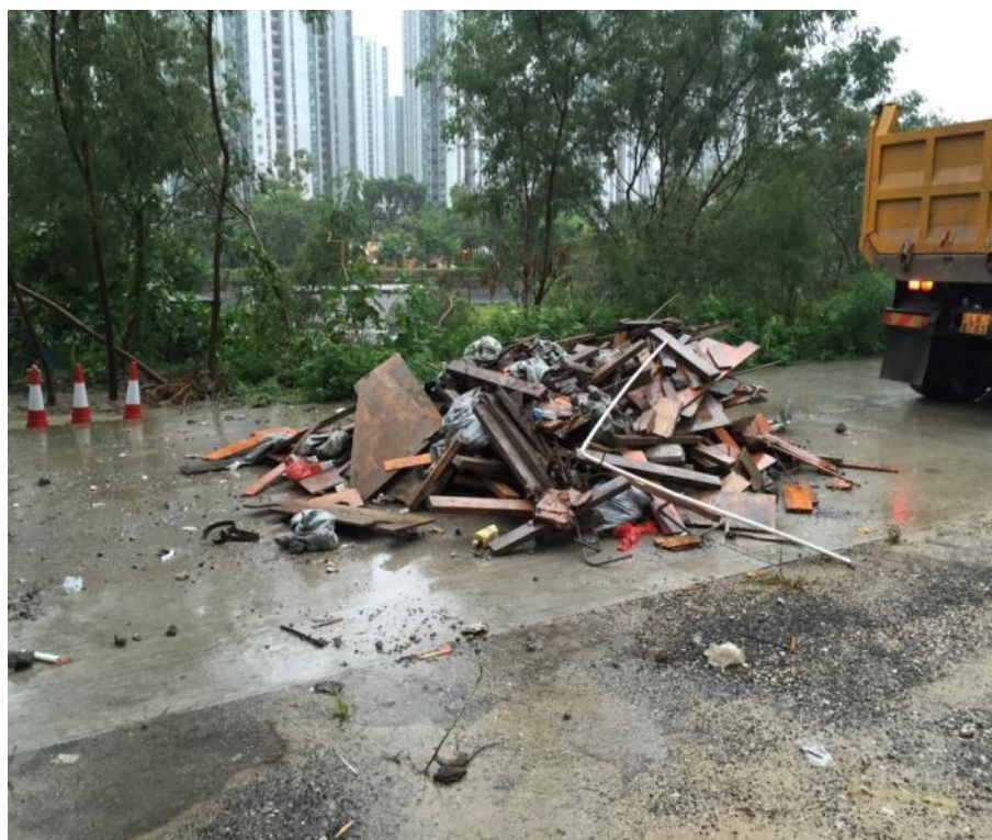
Photo A6: Debris from Site C (II)
