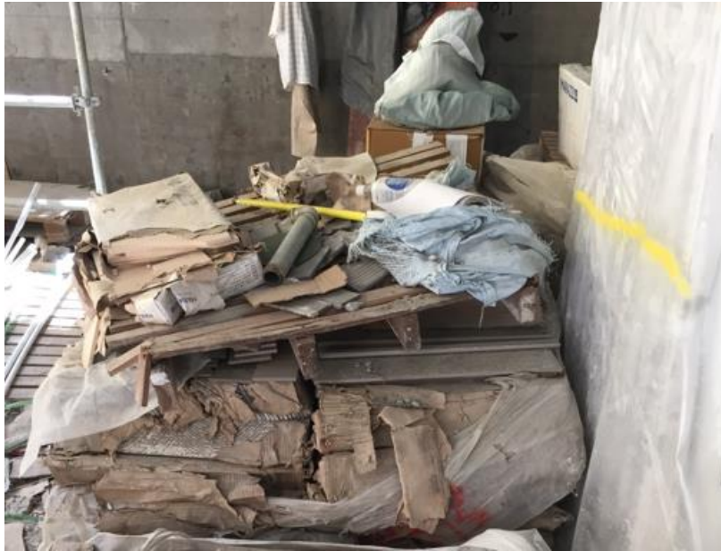
Photo 17: Construction Wastes Noted in a Working Area (1)
