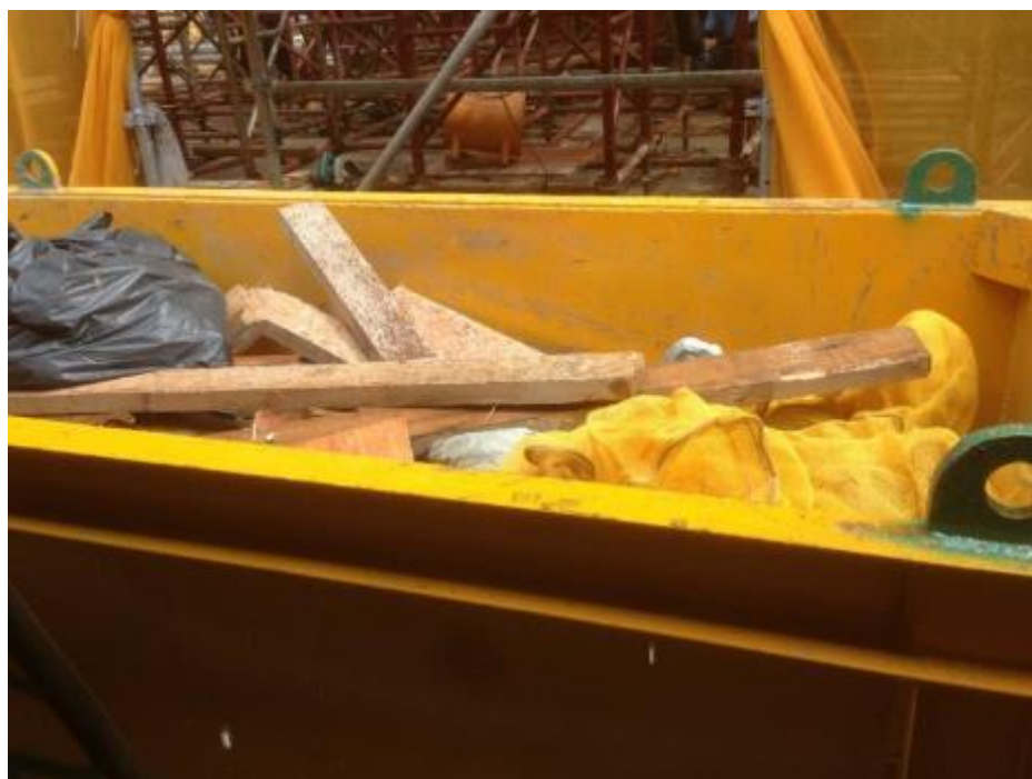
Photo 84: Contents of Construction Waste in Skip B (Mainly Consisting of Nylon Net, Timber etc.)
