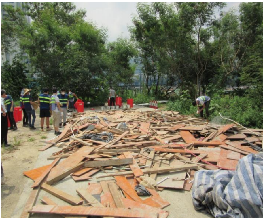
Photo A10: Division of Debris into 4 Parts (II)
