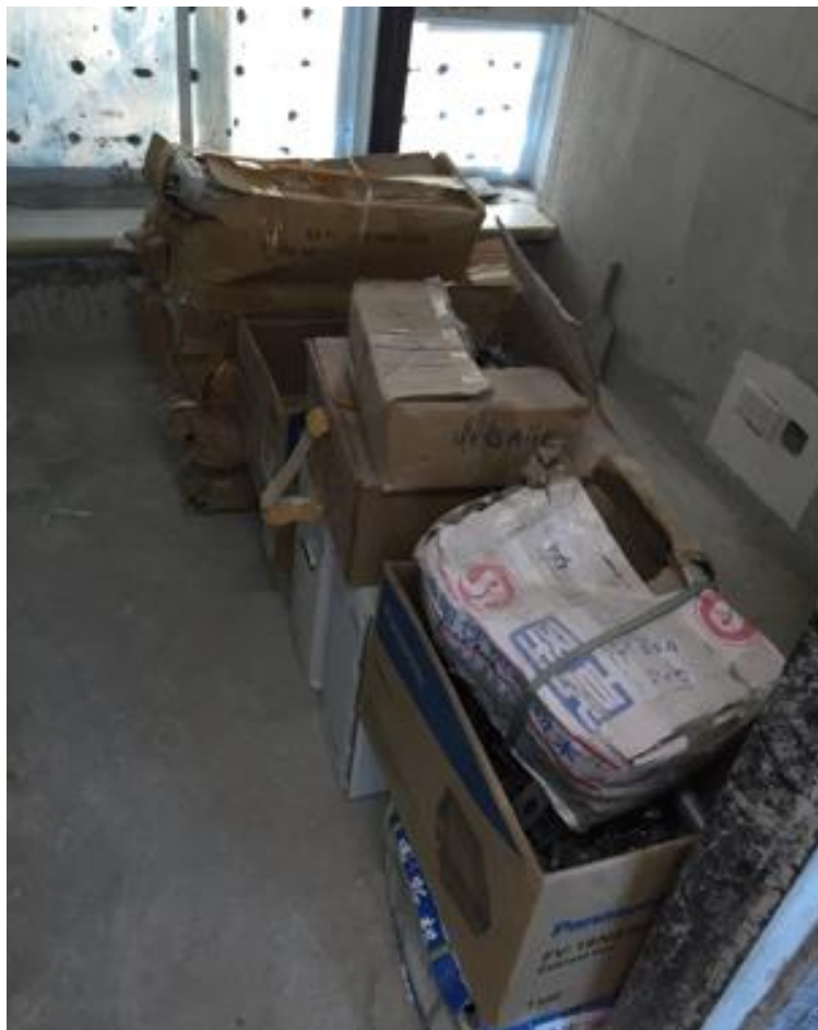
Photo 26: Packaging Wastes in a Working Area of Installing Sanitary Fittings
