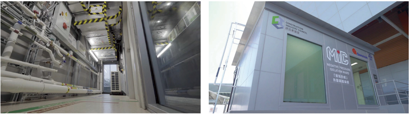
Figure 1.8 Prefabricated plant room modules for a negative pressure isolation ward (Courtesy of Gammon Construction Limited)
