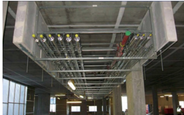
Figure 3.8 Horizontal module integrated with partition wall (Courtesy of BYME Engineering (H.K.) Ltd.)
