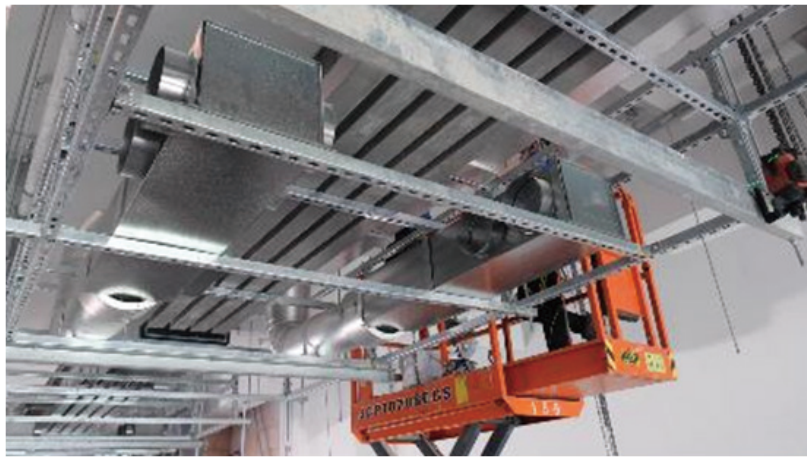
Figure 2.10 Installation of MEP modules and components onsite (Courtesy of FSE Engineering Group Ltd.)
