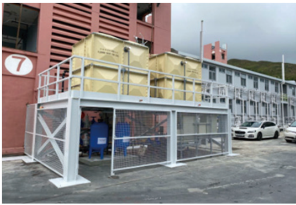
(a) Pump room modules
