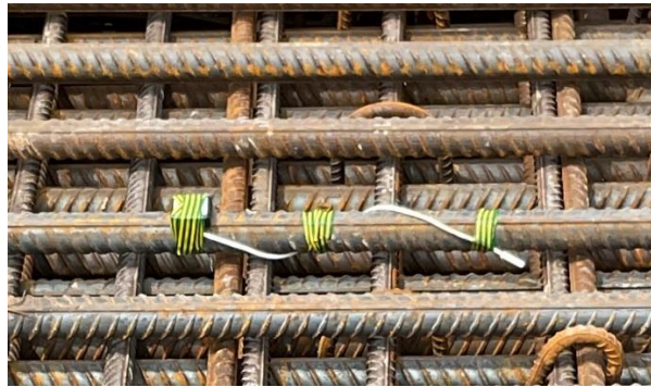
Figure 3. Example of sensor installation with temperature sensor tip not in contact with reinforcement
