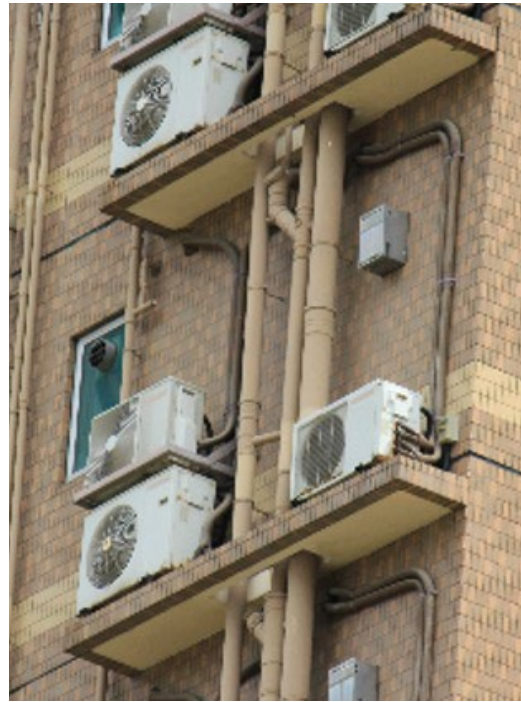
Figure 3 No safe access for air-conditioning maintenance
