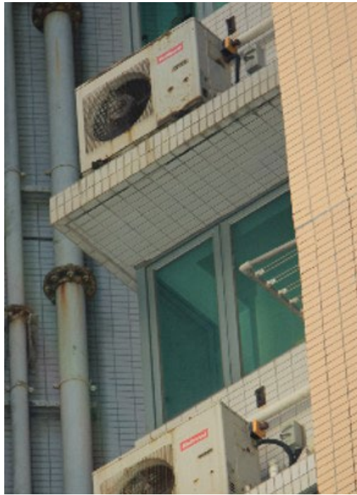
Figure 9 Anchorage point installed in a residential building (Source: Yam et al. , 2007)
