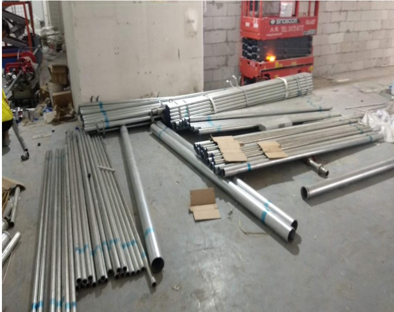
Traditional G.I. Pipe work and fittings need occupies a larger space
