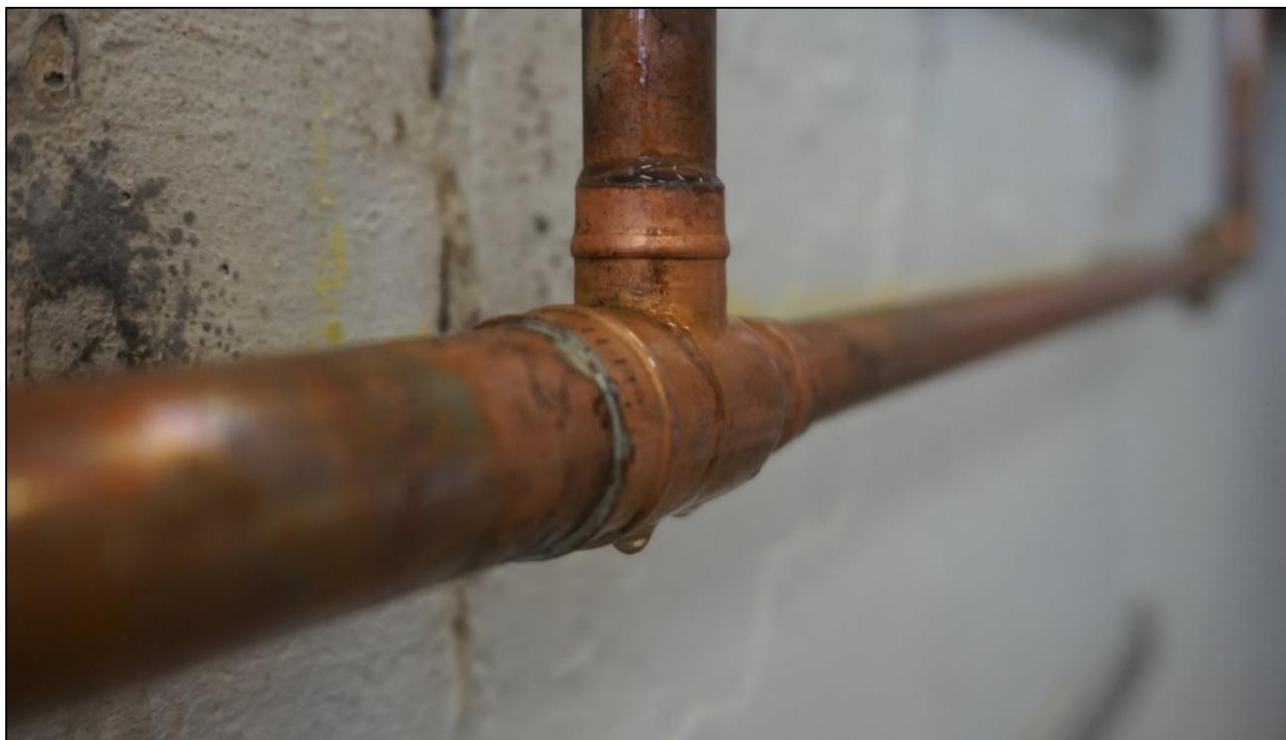
SOLDERING JOINT LEAKGE.
