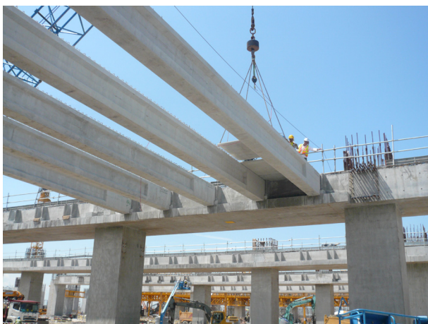
Figure 13 MECHANISED – Subsequent floor construction: Precast I beams precisely located by side restraints and precisely cast on sides of in-situ main beams, still visible on the far left; precast floor slabs being placed from overhead on top of the I beams, necessitating their precise location by the side restraints
