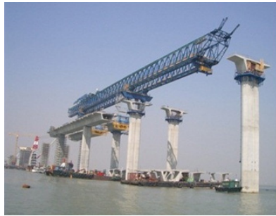
Figure 2 Shenzhen Bay, Deep Bay Link Bridge: Launching gantry used to erect 250 ton precast concrete, bridge deck segment
