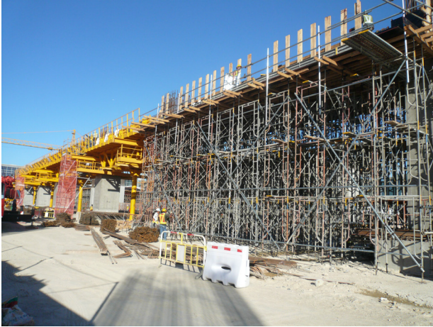
Figure 8 TRADITIONAL – Untidy construction: Wall of scaffold blocking site access; intensive working at height and excessive risk of falling from height; numerous levels of boarded access of dubious integrity; potential for falling of loose materials during erection, dismantling or storage at height
