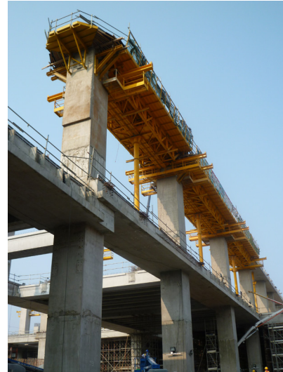
Figure 10 MECHANISED – Multilevel beam construction: Integrated, safe access inside the platform between the columns, for safe working at height; steel formed concrete beams, precisely shaped with high quality finish
