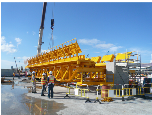
Figure 21 Airport Cargo Handling and Passenger Terminals: Prototype relocated to Hong Kong for training, safely at ground level
