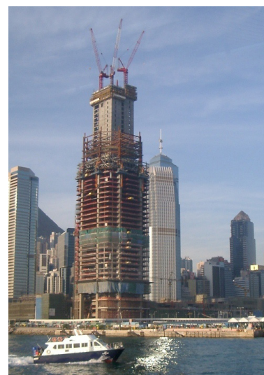
Figure 6 Example of jumpform used in the construction of building core for IFC2
