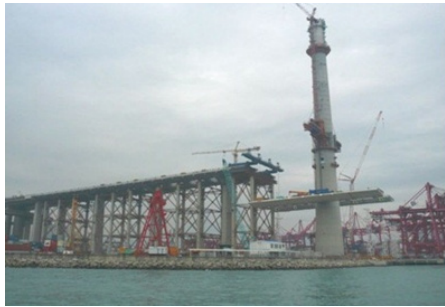
Figure 1 Stonecutters Bridge: Strand jacks used to lift 4,000 ton prefabricated deck from ground level, up to 80 meters and skidding horizontally into the final position
