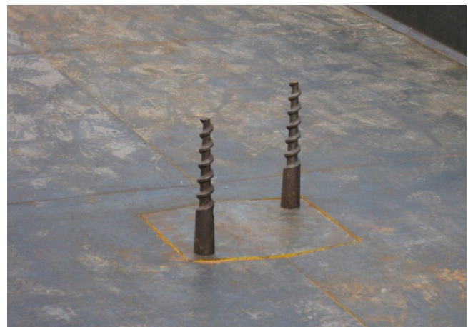
Figure 25 A pair of recoverable anchor screws bolted to steel form ready for concreting
