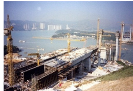
Figure 3 Kap Shui Mun Bridge: Incremental launching of concrete deck, produced in two stage casting bed
