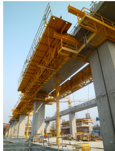
Figure 11 MECHANISED – Preparation for relocation of platforms: Platforms rolled out underneath beam, ready for craning to next beam; central prop remaining to provide support to beam until it has gained sufficient strength to become self supporting
