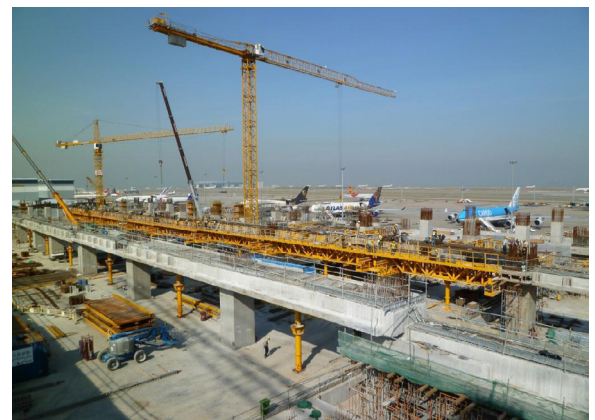
Figure 7 Overview of construction site showing (a) Foreground – Completed multi-span beam with temporary support props (Yellow colour); (b) Background – Platforms in position for the construction of the next beam (Yellow colour)
