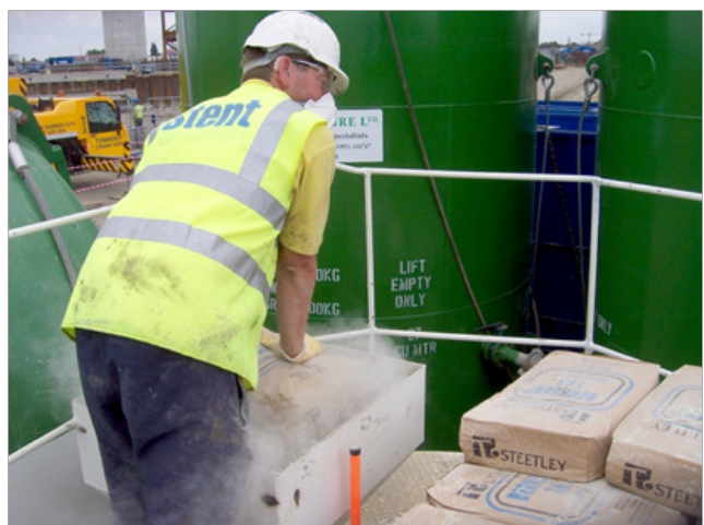
Figure 2 A construction worker wearing a dust mask when breaking paper bags containing bentonite clay powder
